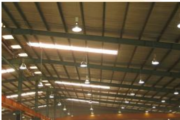
Highbay lamp- factory
